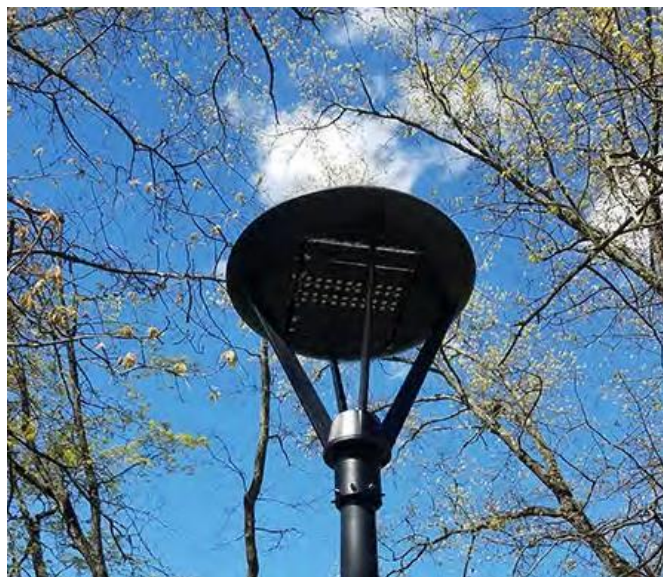
Figure 38. Full cutoff, downward facing light fixture. This parking lot lamp provides light powered by solar cells on the top of the fixture.
