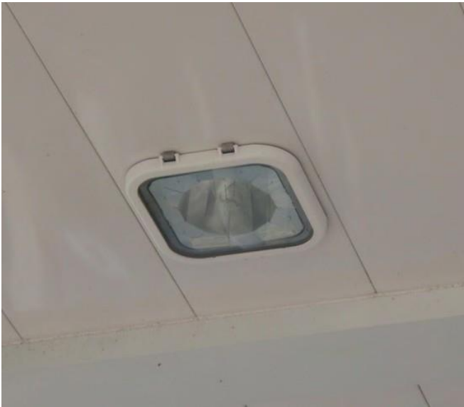
Figure 39. Gas station canopy light. This recessed light in a gas station canopy is ideal because it focuses the light downward and reduces glare to passing motorists.
